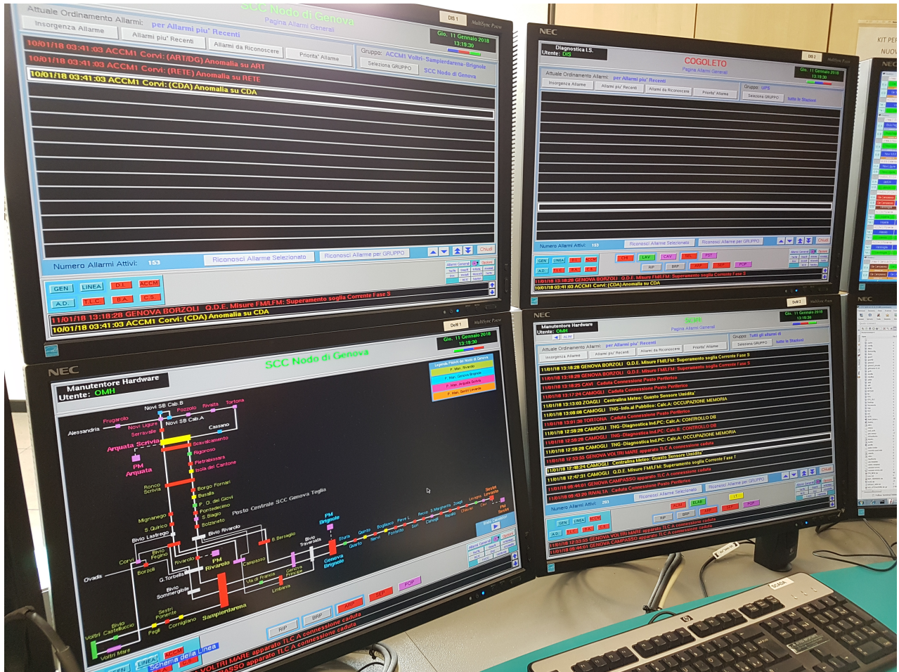
Figure 4: Cross-Scenario 1: Parts of the working station of an asset manager. The lower left monitor shows an overview of an area displaying alarms generated at various train-stations. The remaining three monitors represent filtered lists of alarms for critical systems. Task 2 targets the topological overview system (lower left).
